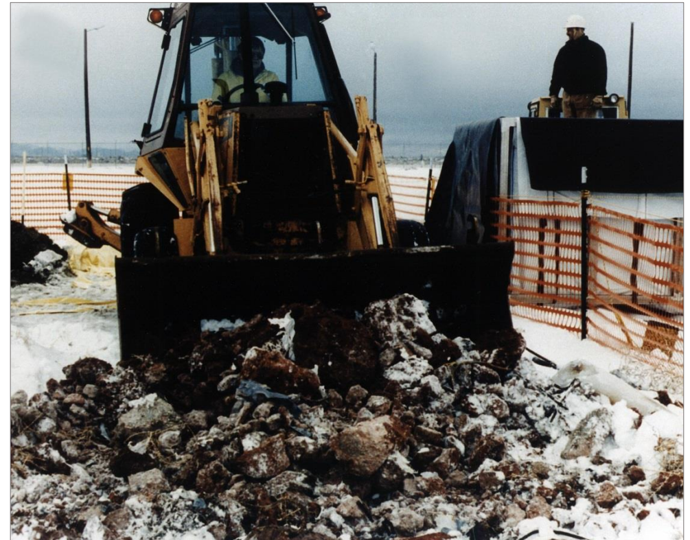
Hauling construction debris to radioactive waste management complex at Idaho National Lab. Photo Courtesy of the Department of Energy.
